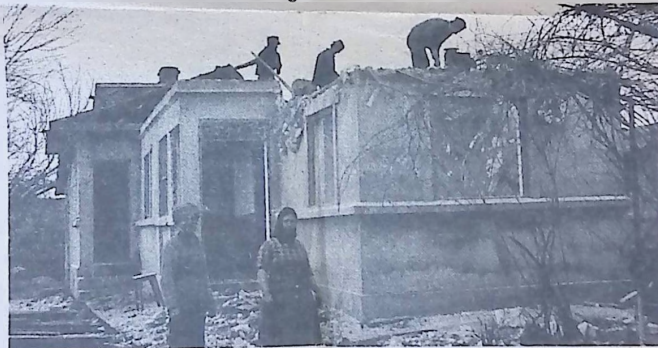
Destruction of a private house in Cornetu, Romania, 1989
