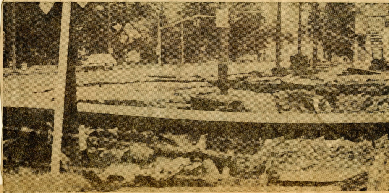
TRACKS SUSPENDED . . . The force of water washed under these railroad tracks between Forty Fort and Kingston
