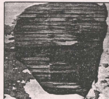
GAPING — A large hole is located in the ceiling of one of the church's rooms
