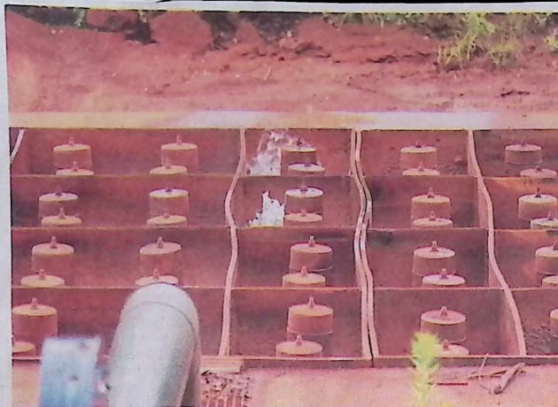
Acid mine discharge flows through a Maelstrom Oxidizer at the Askam Oxidation treatment center on Nanticoke Creek. The water surging up from abandoned mines is packed with iron-oxide, which is essentially rust.
