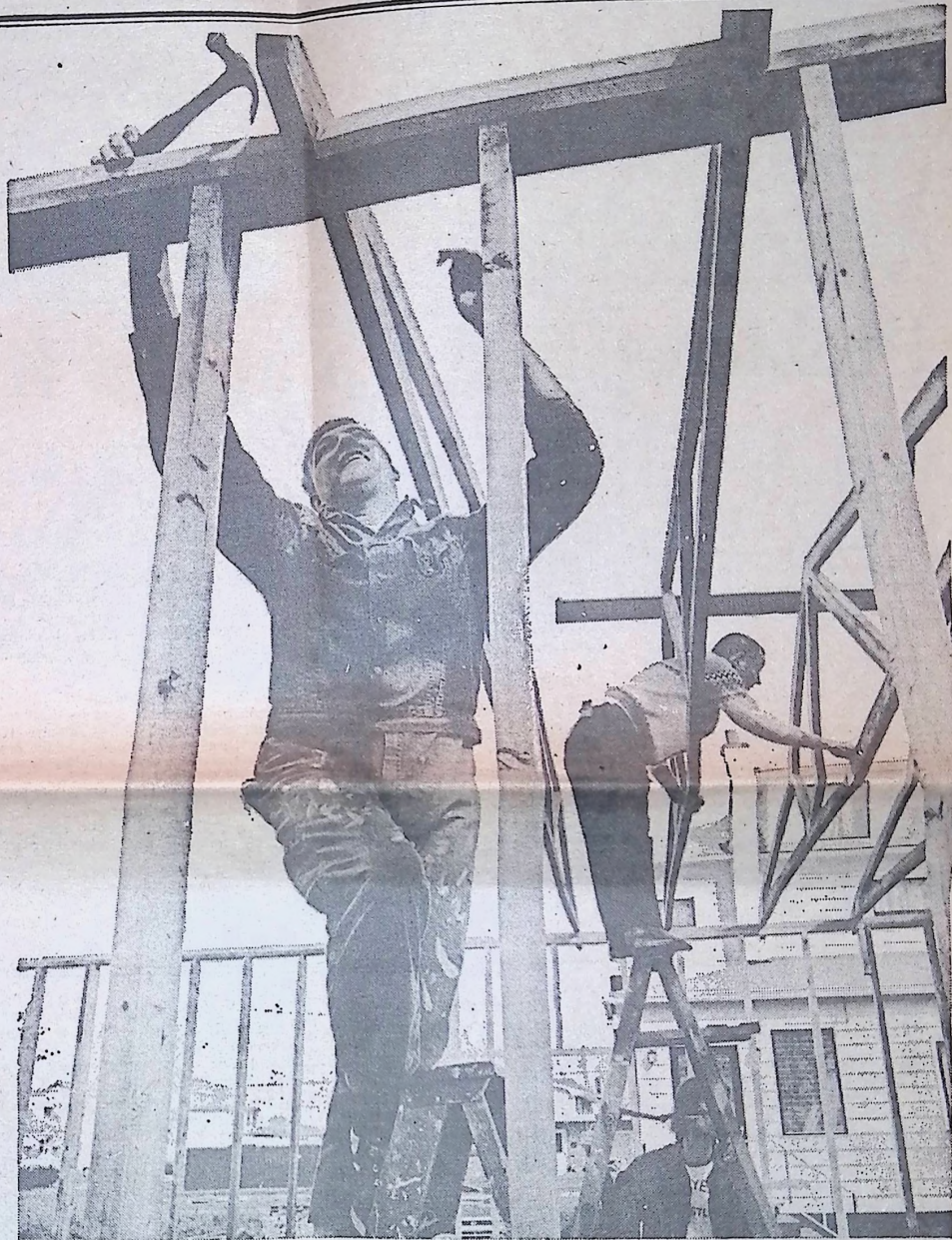
Charles Rupert is still repairing his property in the flood area
