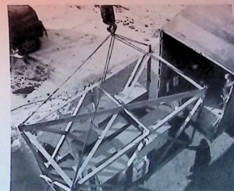
• Top view of the "Crane Cage" shows its sturdy construction and highly diversified usage.
