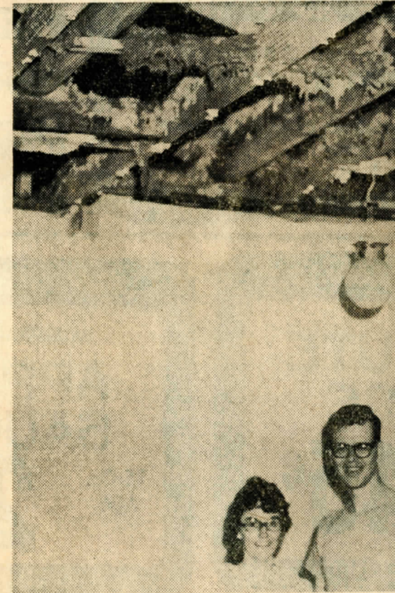
BREACHED AND CRACKED —Deep cracks and breaches in the Gateway Apartments, where an approximate 150-foot-long a Wyoming Valley Sanitary Authority pumping station was seen on top of the two-story apartment buildings had of the flood waters. A Times-Leader Evening News was undermined
