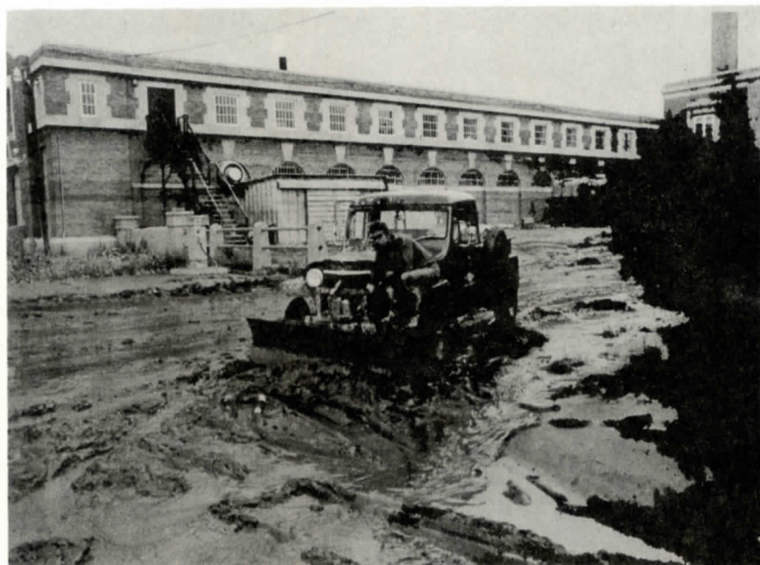
KINGSTON ARMORY...CLEAN-UP OPERATIONS AT ONE OF THE NATIONAL GUARD FACILITIES HIT BY THE FLOOD.
