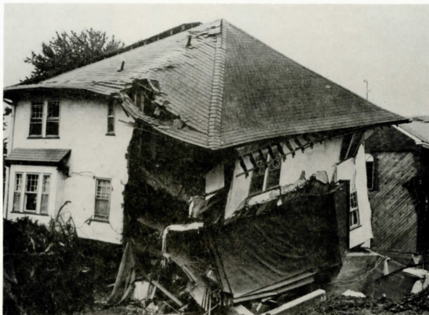
WILKES-BARRE...ONE OF THE MANY HOMES DESTROYED BY FLOOD WATERS.
